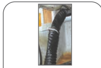
Crushed vent ducting, will impede proper and safe venting of fumes. Replace damaged duct
